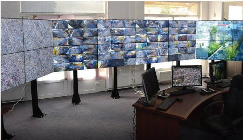
RADWIN radios transmit high-quality video to Police control center
